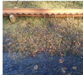
Figure 12 Near-surface irrigation with a labyrinth weir, producing a lateral inflow to the swale.
