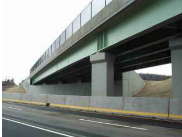
Figure 2.7 Bridge S.R. 0031 over PA Turnpike (Reproduced from Internet) (Spans: 161 ft each span, Skew: 70 degrees)
