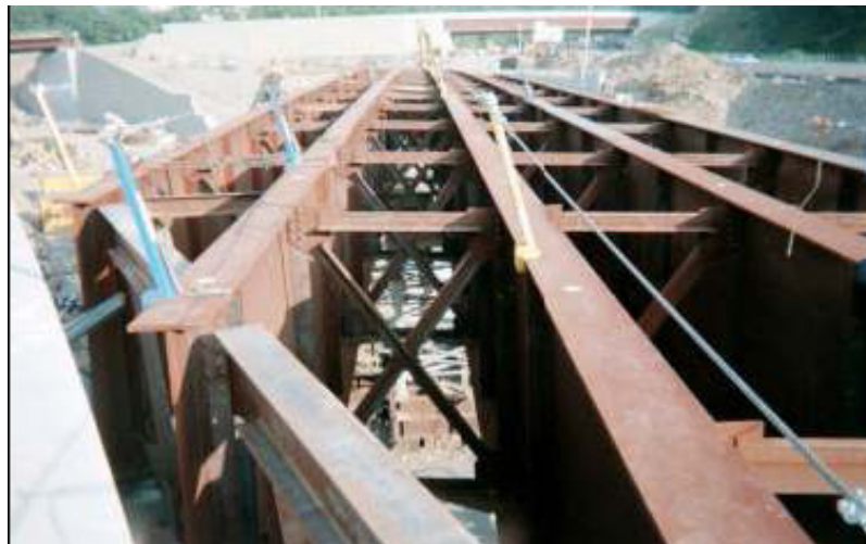
Figure 2.8 Bridge I-87 NB Connectors over I-287 EB (Reproduced from Internet) (Span: 265 ft, Skew: 65 degrees)
