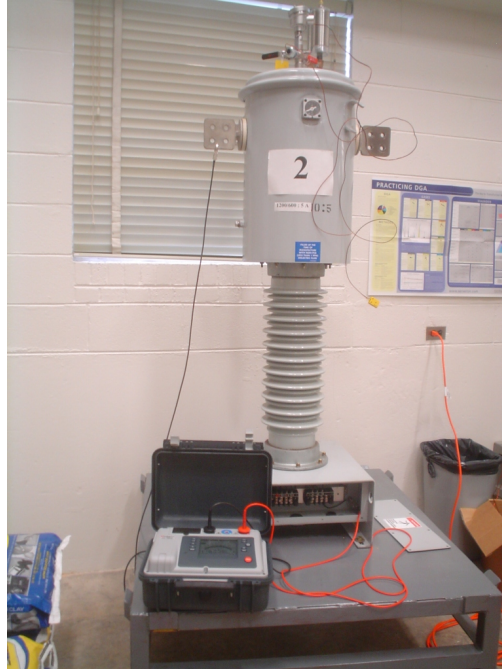
Fig. 156. DC Test carried out on CT2 using the Digital Insulation Tester
