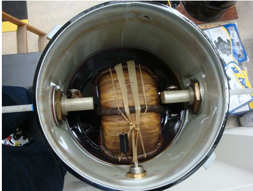
Fig. 113. CT3 Dissection – Draining Oil, observed primary, secondary, and core insulation
