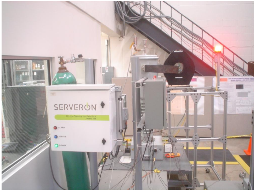
Fig. 161. DGA monitoring system - As installed in the HV/HC Lab CH-103
