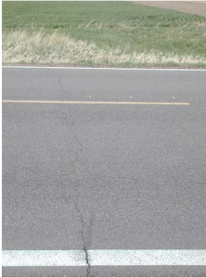
Figure 4.4 Visible transverse cracks on K-25 project
