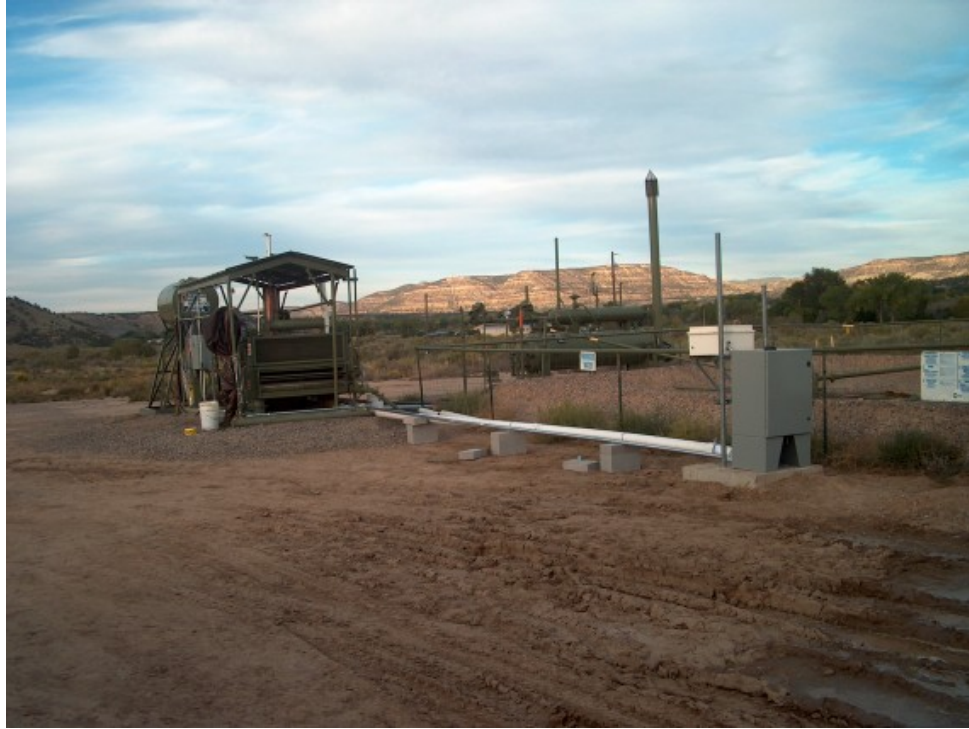
Figure D.1 Engine 1 picture showing the instrumentation box
