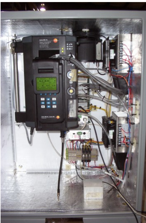
Figure D.6 Inside the Instrumentation box showing the portable analyzer
