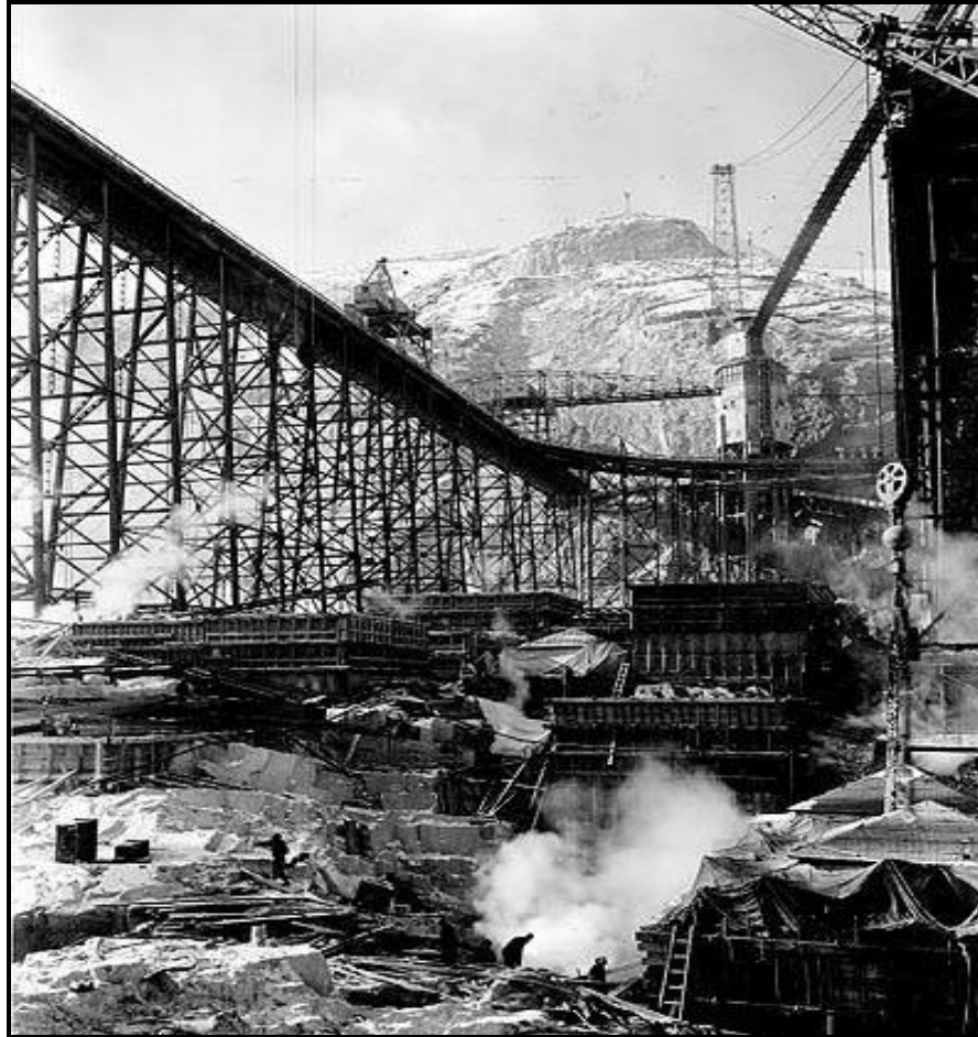
Figure 13. Laborers Placing Concrete with Cranes and Trestles, Grand Coulee Dam Construction Site, 1936. University of Washington, Special Collections. No. DAM129.
