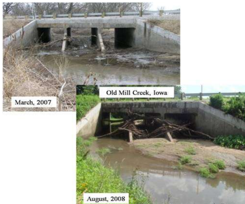
Figure 1.2 Typical sedimentation pattern at a culvert in Iowa
