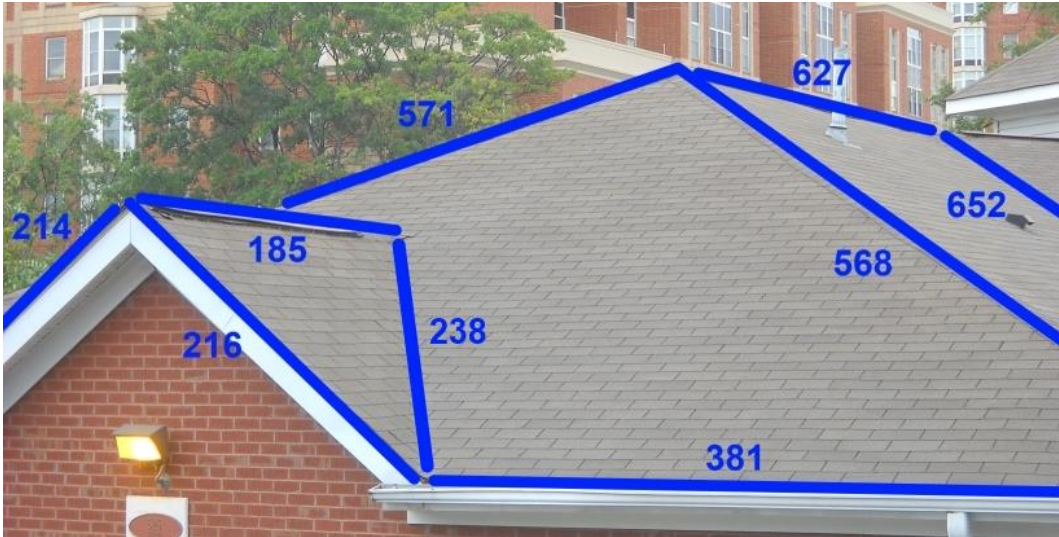
Figure 4.25: Extracted measurements for the second complex roof. The numbers and lines have been printed manually on an image from the roof structure.
