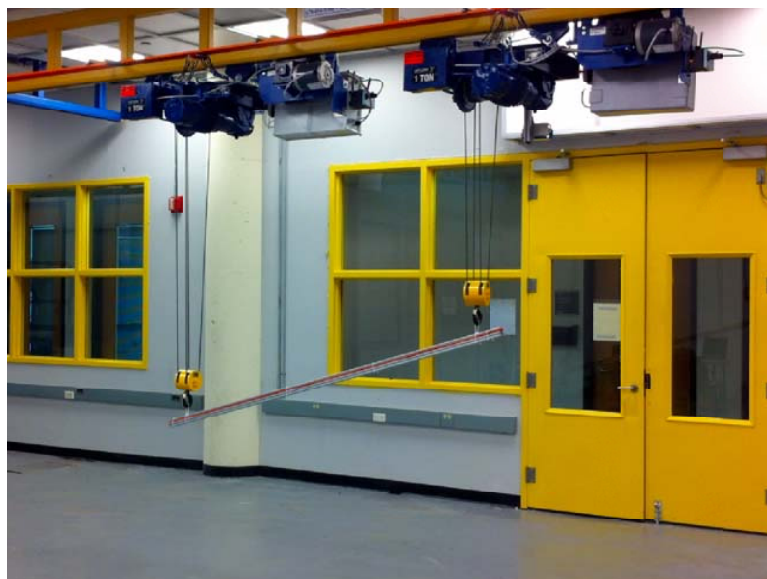
Figure 7.1: Dual-Hoist Bridge Crane
