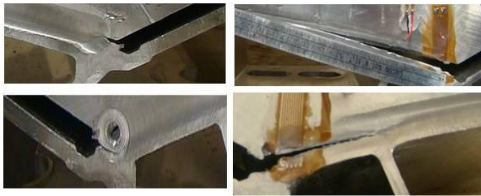
Figure 7.22: FSW cracks at 5 kph and 10 kph energies (left to right).
