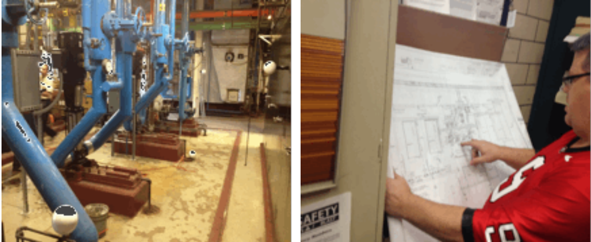
Figure 10: A typical working environment of a HVAC Technician in a healthcare facility (Grady Hospital, Atlanta, GA, USA)
