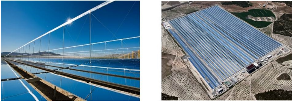
Figure 1.7: LFR collector field at Puerto Errado 2 Thermosolar power plant in Calasparra (Murcia, Spain) [10].
