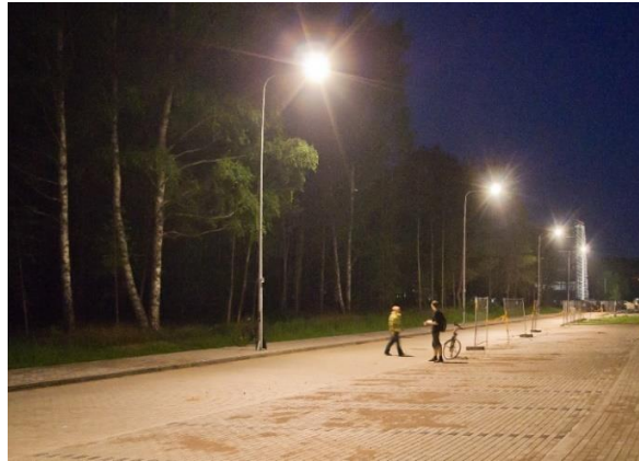
Fig. 4.1. Photograph of the lighting installation at Vilnius University campus [P13].
