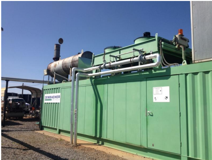
Figure 6. Jenbacher Engine 2 with installed heat exchanger.
