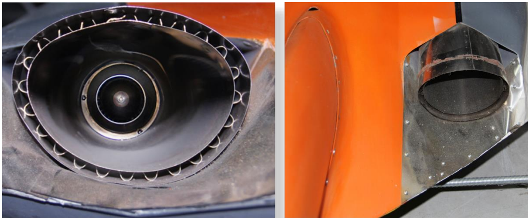
FIGURE 46 - EXHAUST OUTLET SHOWING CUSTOM DOUBLE WALLED THRUST TUBE (LEFT) AND STAINLESS STEEL FLASHING ON STRUCTURE TO PREVENT HEAT DAMAGE TO STRUCTURE (RIGHT)
