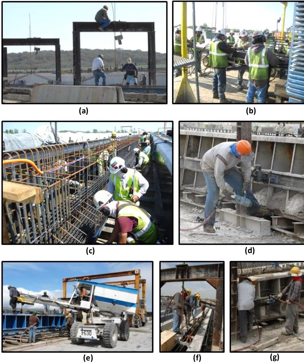
Figure 3-5: Fabrication of a typical specimen: (a) harping of strands, (b) tensioning of strands, (c) placement of mild reinforcement, (d) installation of side forms, (e) concrete placement, (f) internal vibration, (g) external vibration
