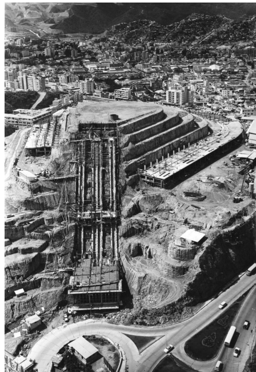
FIGURE 11.27 Helicoid’s earthwork, ca. 1957 (almost same viewpoint than fig. 11.28 ). The structure to receive the inclined elevators was quite advanced, as well as some section of the ramp. Source: Dirk Bornhorst Archive.
