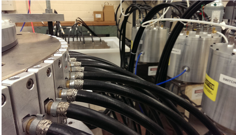
Figure 3.8: Left: collet plates secure cables to triplate perimeter. Right: capacitor bank modules 6, 7, and 8. Background: charge dump tank with charge cables.
