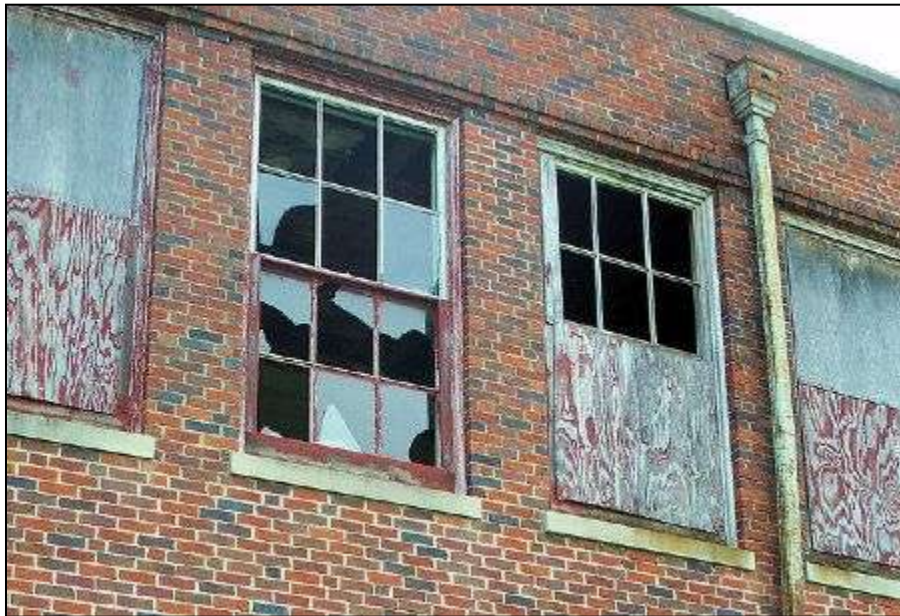
Photograph 12: Buildings with broken windows soon invite further vandalism and can lead to aggressive and violent behavior in surrounding areas. A building left with broken windows indicates that little care or attention is directed toward the building or area around it.
