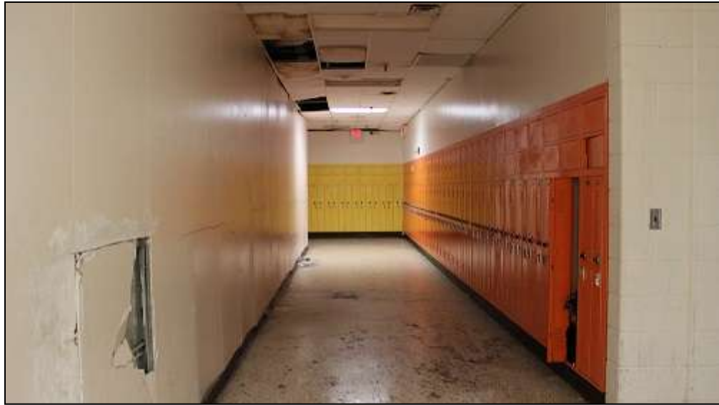
Photograph 16: Broken walls, stained ceiling, dirty floors, dim lighting, and confined design all make this hallway unappealing and a target for further neglect and destruction.
