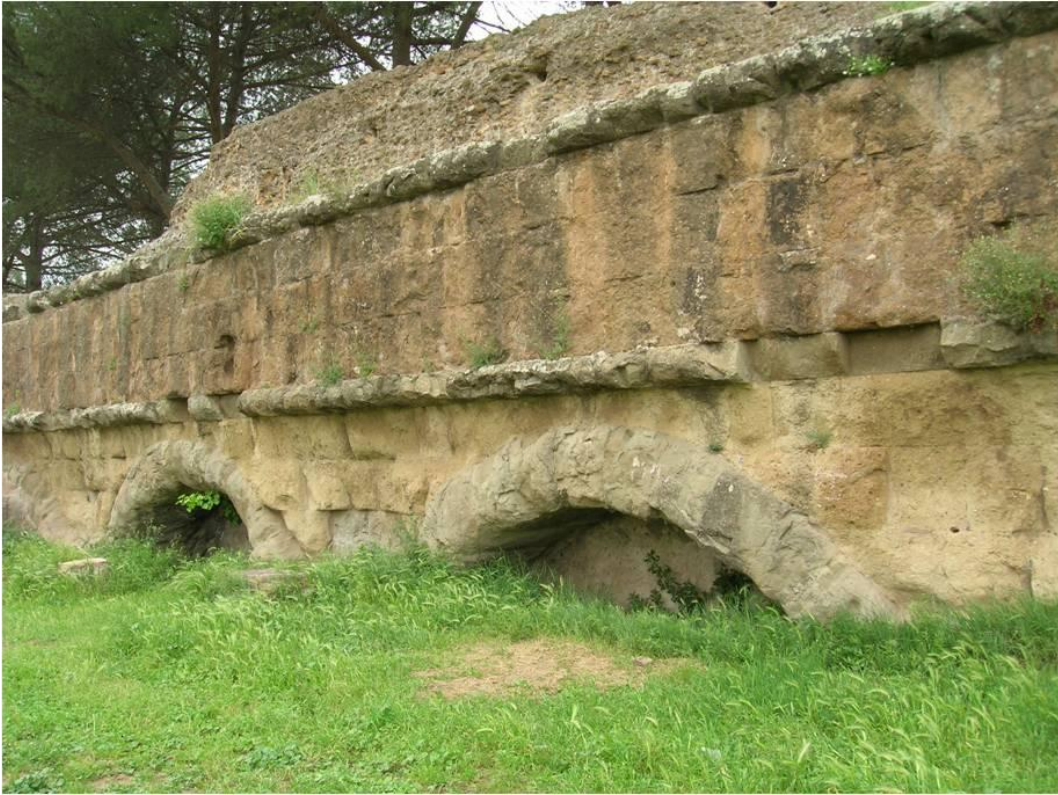
Figure 3.8 A section of the Aqua Marcia for comparison. Please note that the Aqua Marcia is in a much poorer state of preservation (Photos Joelle L. Lardi 2009)
