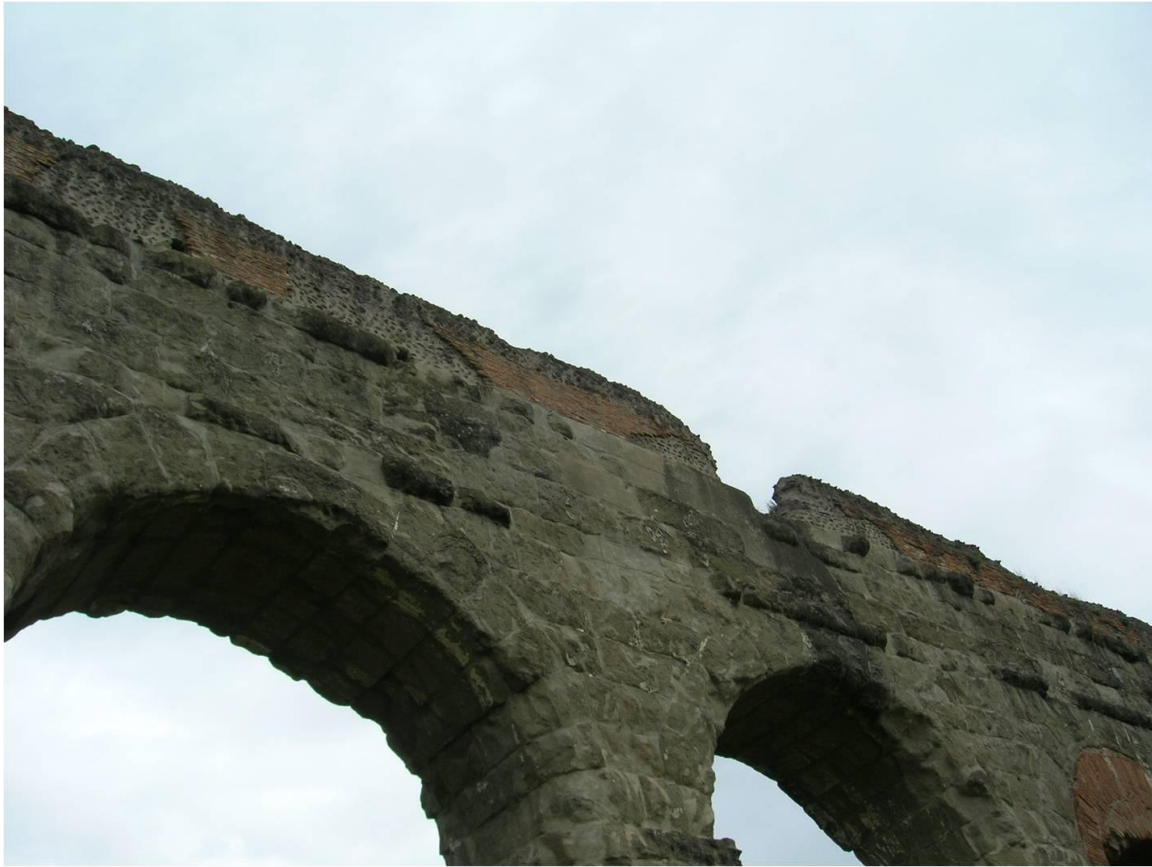
Figure 3.2 The Anio Novus specus is clearly distinguishable here by its different building material, brick and concrete. (Photo Joelle L. Lardi 2009)
