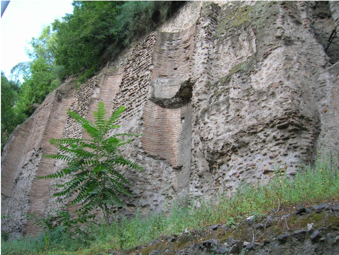
Figure 5.18 Part of the articulated façade of the Celian Nymphaeum (photo J.L. Lardi 2008)
