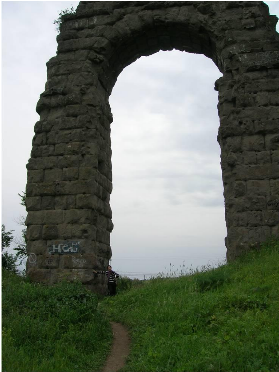
Fig. 3.7 Individual arch of the Aqua Claudia showing size and texture of individual building stones. Note the person for scale. (Photo Joelle L. Lardi 2009)
