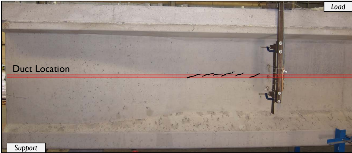
(A) Localized diagonal cracks along post-tensioning duct occur at shear force ( V_{LC} )
