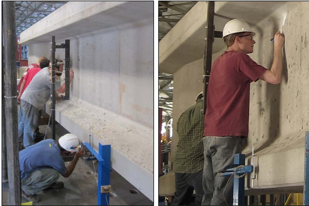
Figure 3-34: Cracks Marked with Felt Tip Marker
