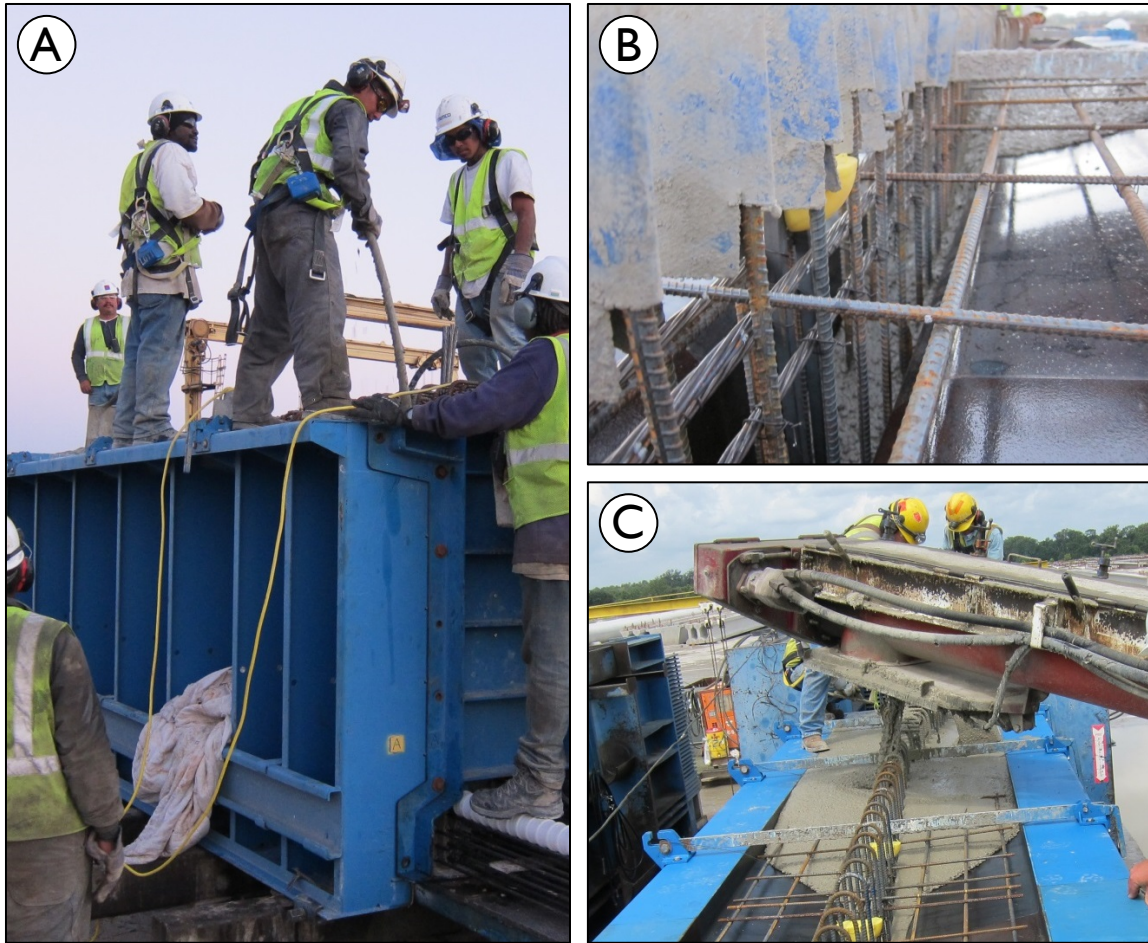
Figure 3-17: Concrete Consolidation (A) “Stinger” Type Vibrators Used within End-Block & (B), (C) Self-Consolidating Concrete Flow
