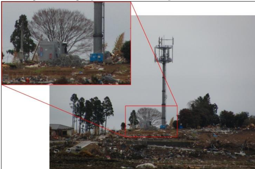
Fig 4.3 A portable genset powering a base station near the town of Saichi [TCLEE 2012].
