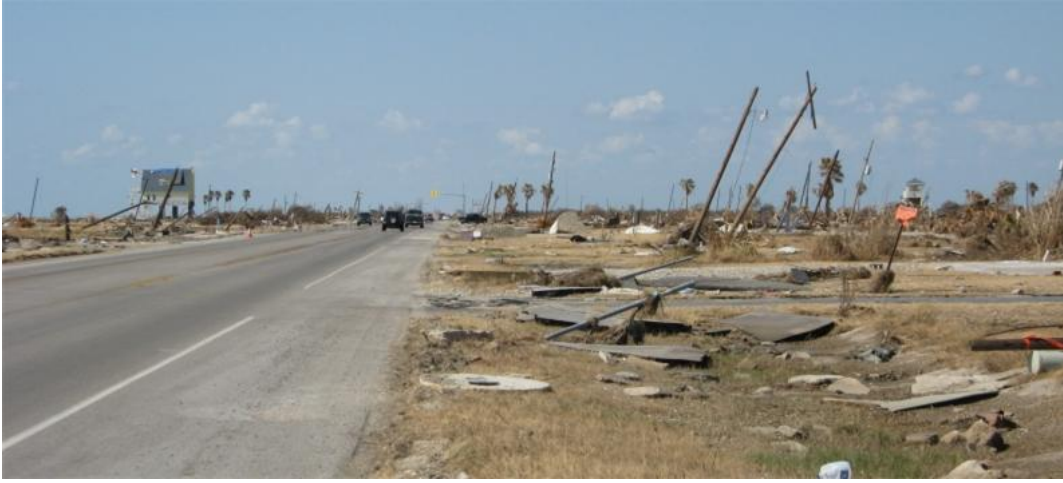
Fig. 2.1. Area where all the power infrastructure was destroyed (Gilchrist, TX).
