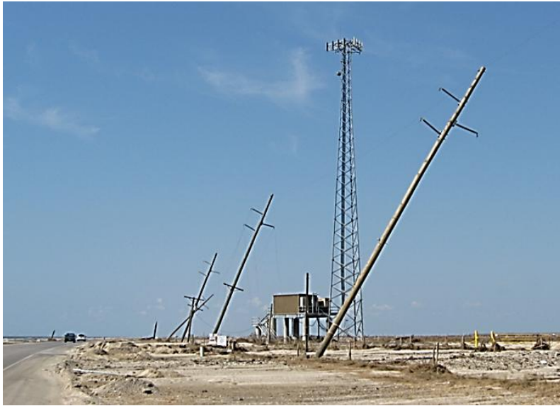
Fig. 1.1 Telecommunication base station after Hurricane Ike 2008.
