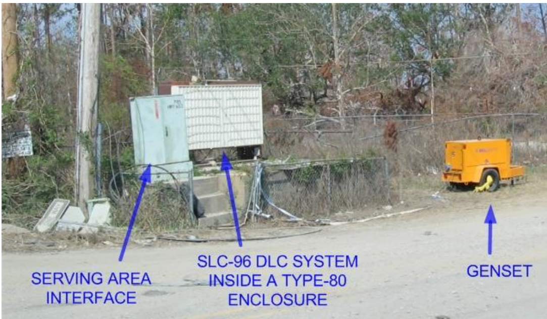
Fig 7.3. DLC system powered by genset after Katrina.
