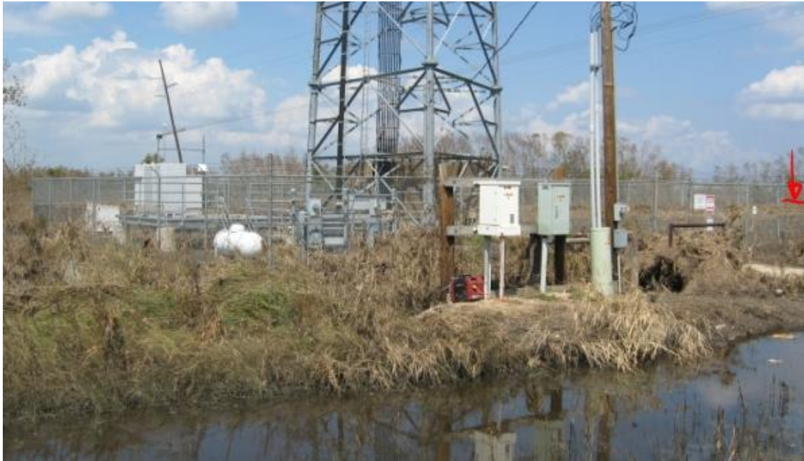
Fig. 7.7 Destroyed Cell site and DLC Hurricane Ike [Kwasinski 2008a]
