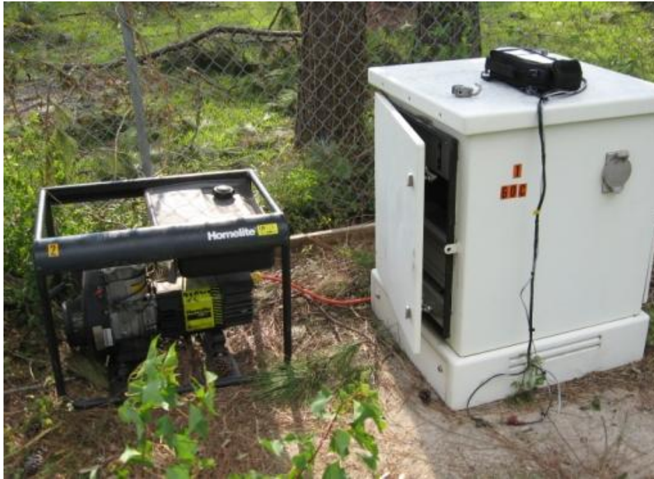
Fig. 7.5. Failed DLC during Hurricane Ike due to loss of power [Kwasinski 2008a]
