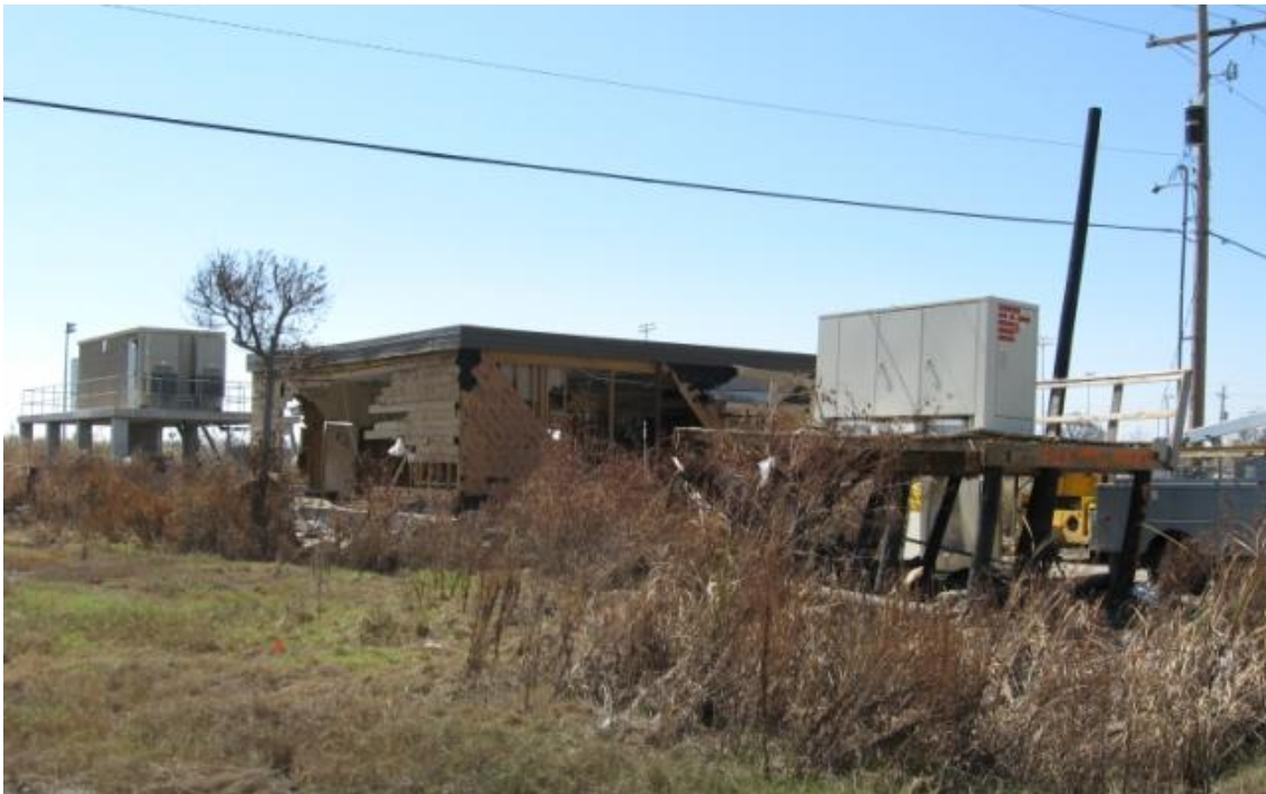
Fig 7.6. Hurricane Ike , Sabine TX, Central office destroyed[Kwasinski 2008a]
