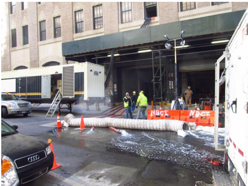
Fig. 7.9. Water being pumped out of the central office in Manhattan after Sandy [Kwasinski 2012a]
