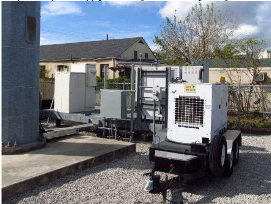
Fig. 4.4 Fuel Cell deployed for DLC after Hurricane Isaac.
