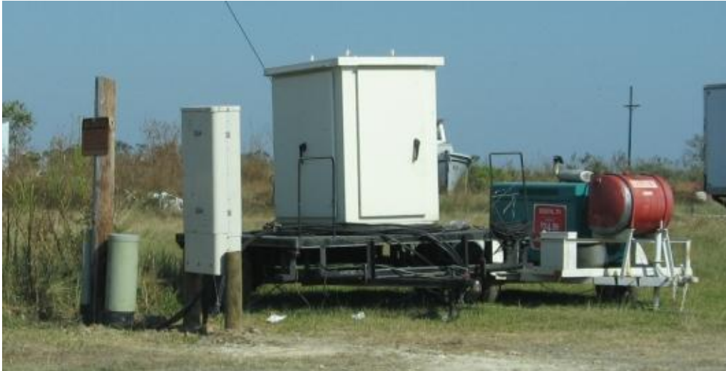
Fig. 4.2 DLC with temporary diesel genset installed after Hurricane Ike.
