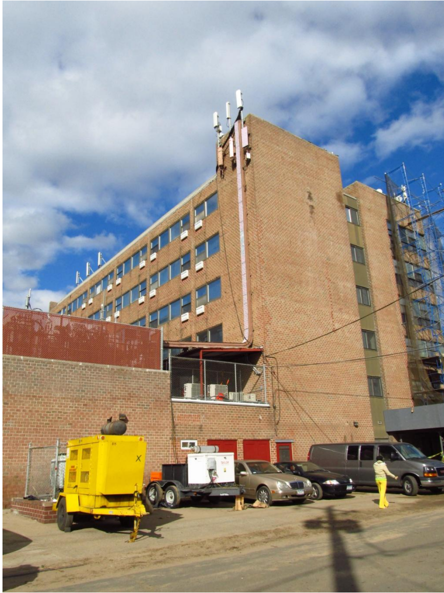
Fig. 7.10. Rooftop cell site in Rockaway Peninsula, New York
