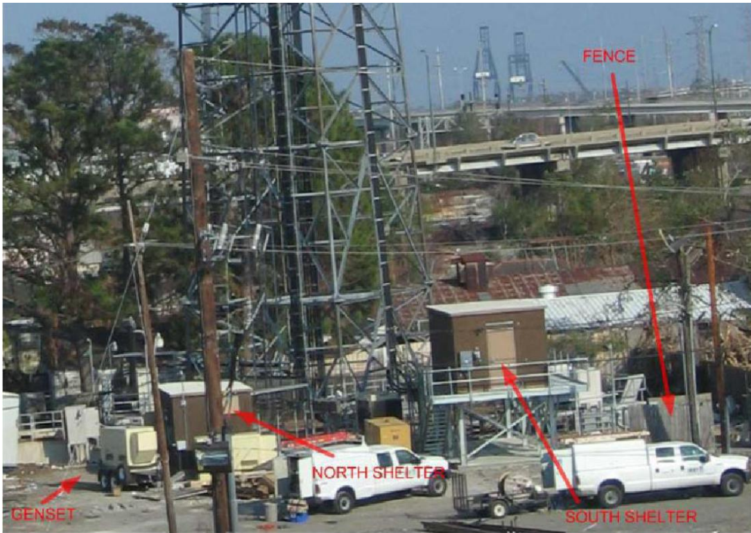
Fig. 7.2. Cell site in New Orleans after Katrina
