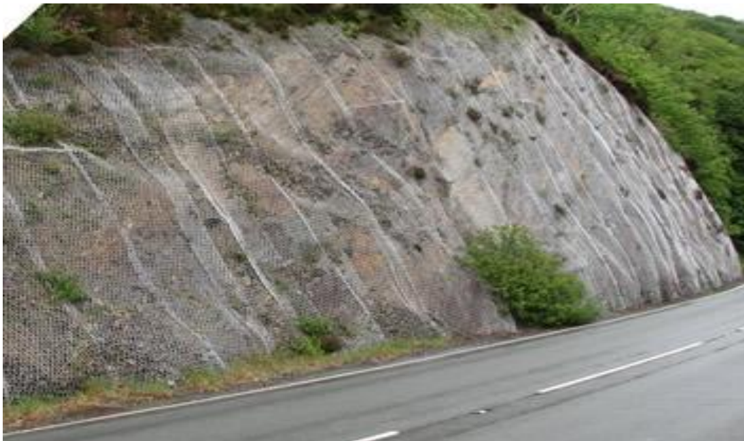
Figure A.6 Example of a Rockfall Location (Hazard)
