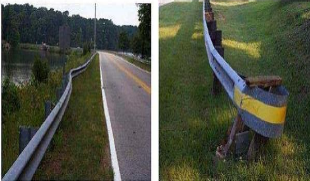
Figure 2.4 Underperforming Guardrails (Kim, et al., 2009)
