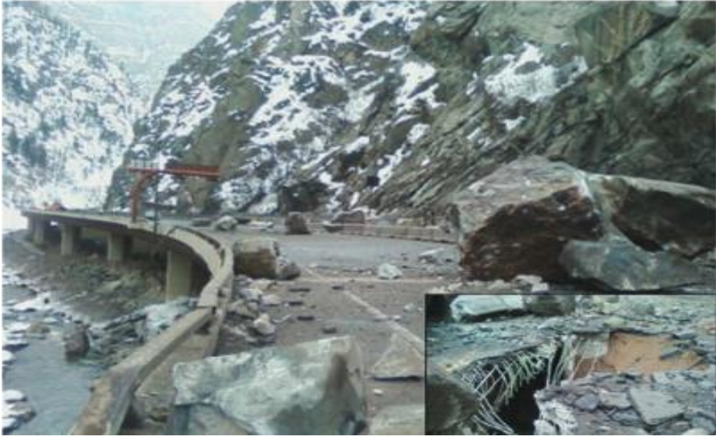
Figure 2.6 Rockfall in Glenwood Canyon, Colorado (Anderson & Rivers, 2013)
