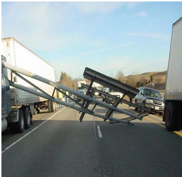
Figure 2.3 A Failed Cantilever Overhead-Sign Structure (Garlich & Thorkildsen, 2005)
