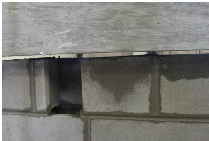
Figure 122: Gap between the top of the infill wall and the RC frame
