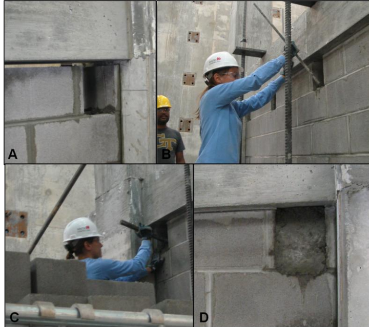
Figure 119: At the top of the masonry wall, (a) face shell of the grouted cell was removed, (b) weak concrete was poured into the 3 courses below, and (c-d) the last course was dry packed
