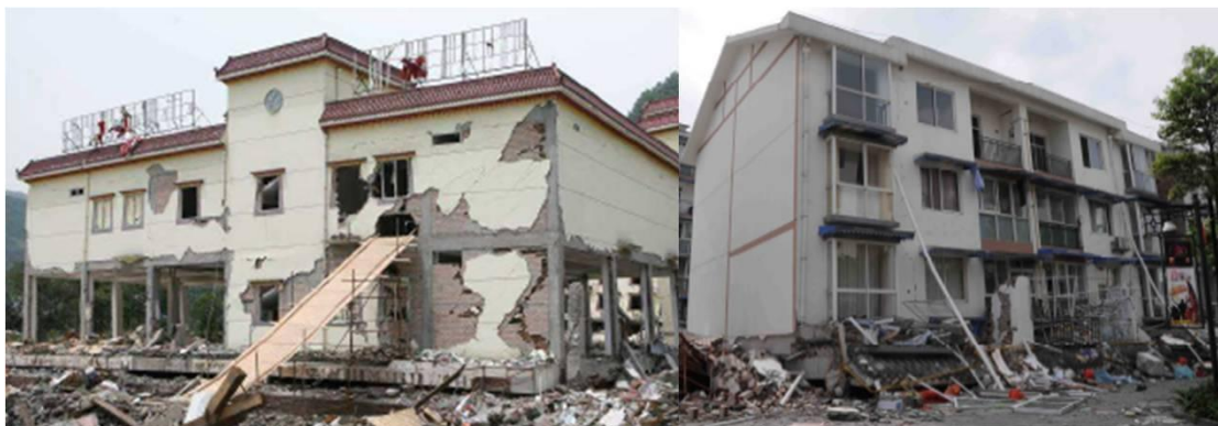
Figure 19: Damage from the Wenchuan earthquake: shear failure and collapse of masonry (left) and collapse of a 5 story building (right) (Li et al. 2008)
