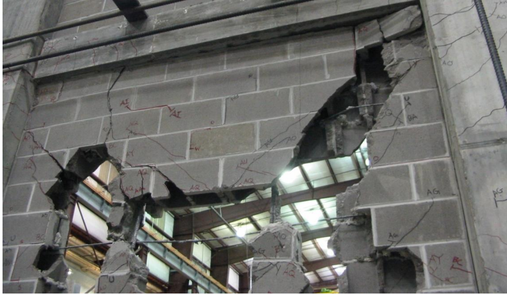
Figure 150: Top section of masonry wall of Frame 2 (connection only at the base) was in danger of out-of-plane collapse by 1.8 inches (45.7 mm) of lateral displacement (1.5% drift).
