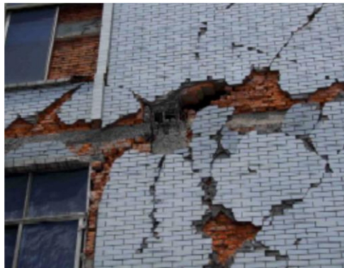
Figure 20: Solid infill which helped prevent building collapse (Li et al. 2008)
