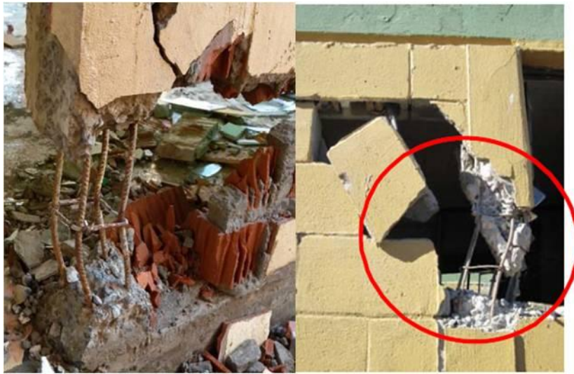
Figure 25: Buckling of rebar at foot of column (left) and shear failure of first story column (right) (Brzev et al. 2010)
