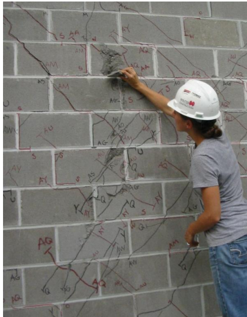
Figure 145: Close up of crushing of the masonry face shells near the diagonal cracks at 0.82 inches (20.8 mm) of lateral displacement (0.683% drift).
