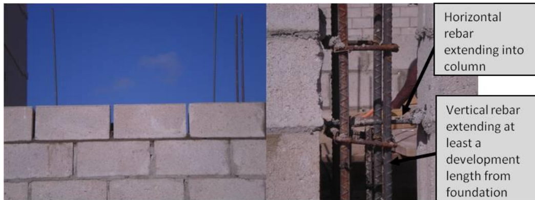
Figure 7: Close up of vertical rebar spacing (left) and rebar connection to column (right)
