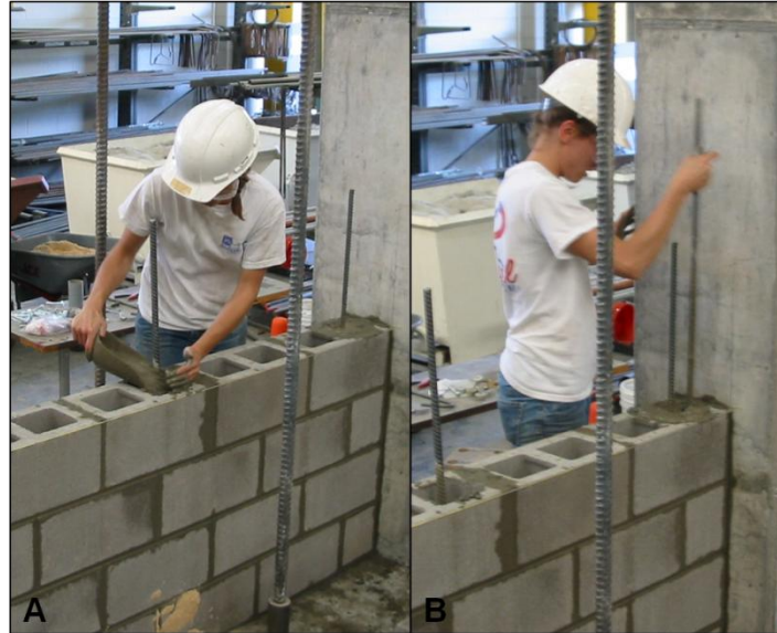
Figure 116: Reinforced cells filled with concrete (a) and consolidated with a rod (b)
