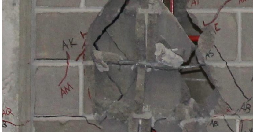
Figure 162: Bending of horizontal reinforcement just past the termination of the dowel bar in the Frame 1
