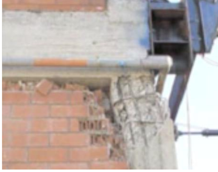
Figure 17: Shear failure due to short-column effect from crushing of masonry at corners (Corte et. al. 2008)
