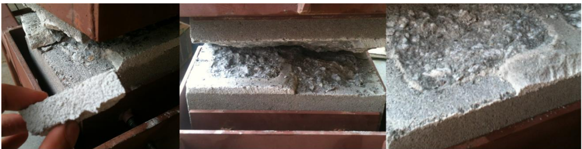
Figure 194: Failures of grouted bed joints
