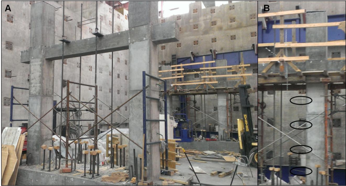
Figure 102: Disassembly of the shoring and formwork (a) and close up of frame with dowel connections (b)
