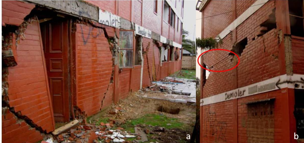
Figure 24: (a) In-plane shear failure of first story (b) Out-of-plane failure of second story (Brzev et al. 2010)
