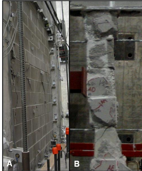
Figure 148: Large portion of masonry face shell (a) fell out of plane and revealed (b) grouted cores with shear cracks in Frame 1 at 1.8 inches (45.7 mm) of lateral displacement (1.5% drift).
