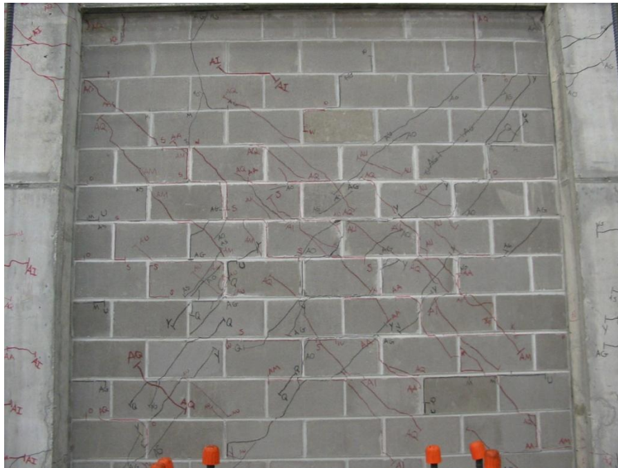
Figure 142: Close up of the masonry wall in Frame 2 (connection only at the base) at 0.58 inches (14.7 mm) of lateral displacement (0.483% drift). The cracks in the experiments are traced in black for the positive cycles and red for the negative cycles.
