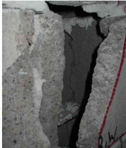
Figure 161: The horizontal reinforcement placed at the center of the unit caused the masonry web to split
