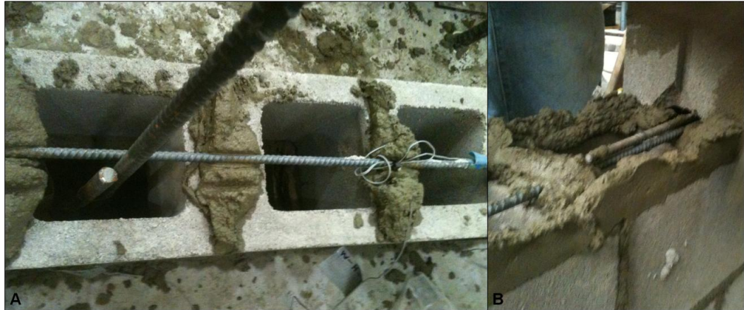
Figure 114: Horizontal reinforcement (a) placed over grouted webs and (b) spliced with dowel bars from columns
