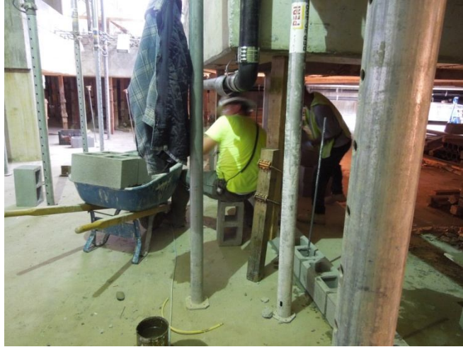
Figure 21- Two laborers carrying block on a wheel barrel and stocking units in the work area.
