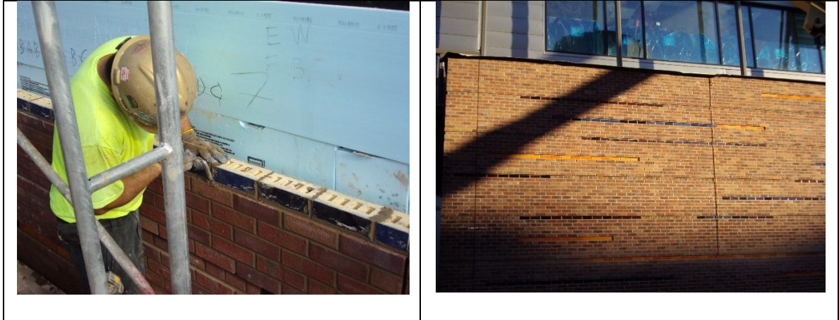
Figure 32a- Mason working on a high quality brick veneer wall; Figure 32b- High quality wall with insertions and color brick
