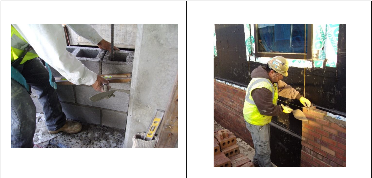
Figure 30a- Mason using the level to build a block wall; Figure 30b – Mason working on a wall with numerous windows
