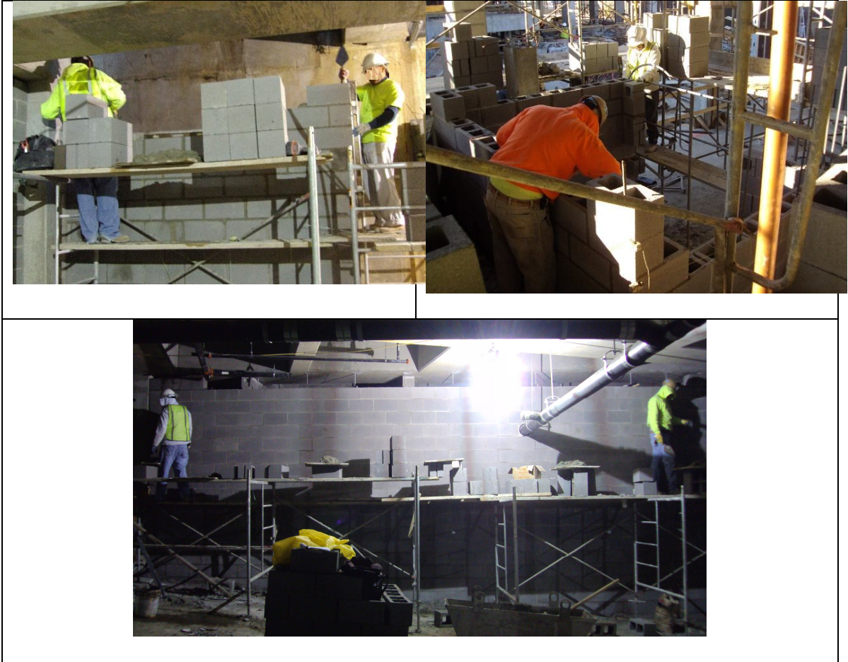
Figures 27a, 27b, 27c,- Masons assigned repeatedly to work together in different wall sections
