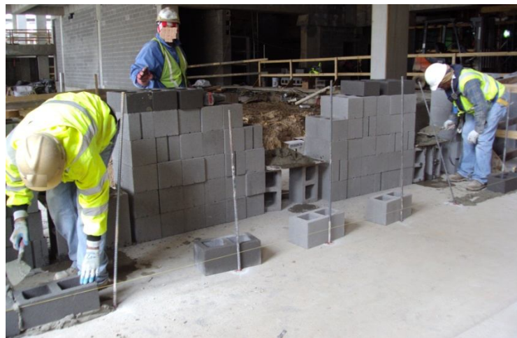
Figure 12- A crew of two masons (front) and one laborer working on a block wall
