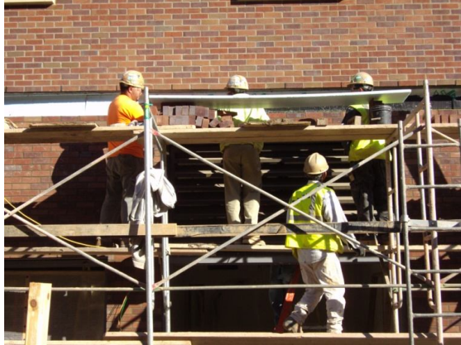
Figure 11- Crew of three masons (top) and one laborer working on a brick veneer wall
