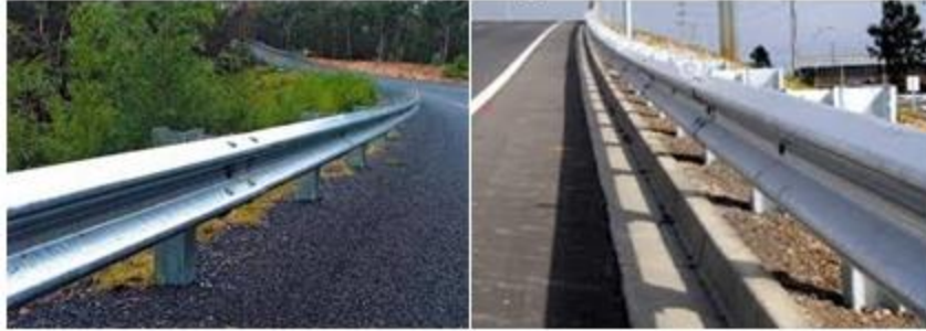
Figure D17 Examples of Roadside Barrier
