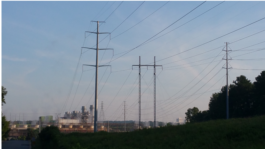
Figure 9: Example of 230 kV high-voltage transmission lines running from Atlanta’s Plant McDonough-Atkinson. From left to right are a double circuit single pole davit arm, single circuit H-frame, and a different double circuit single pole davit arm.
