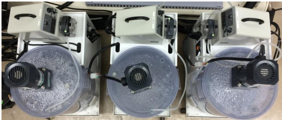
Figure 2.14: Three slurry/DI water tanks of the APD-800.
