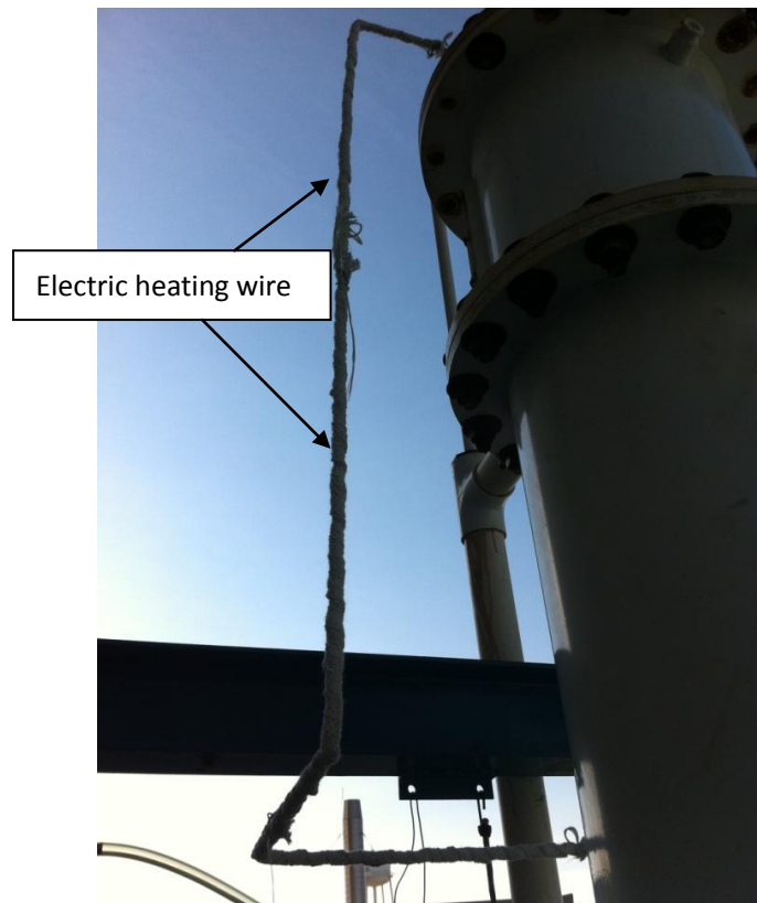
Figure A.7: Heated sample line (outside)
