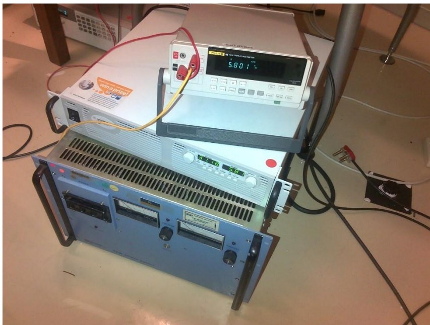
Figure A.11. Electrical equipment used to power up the lamps
