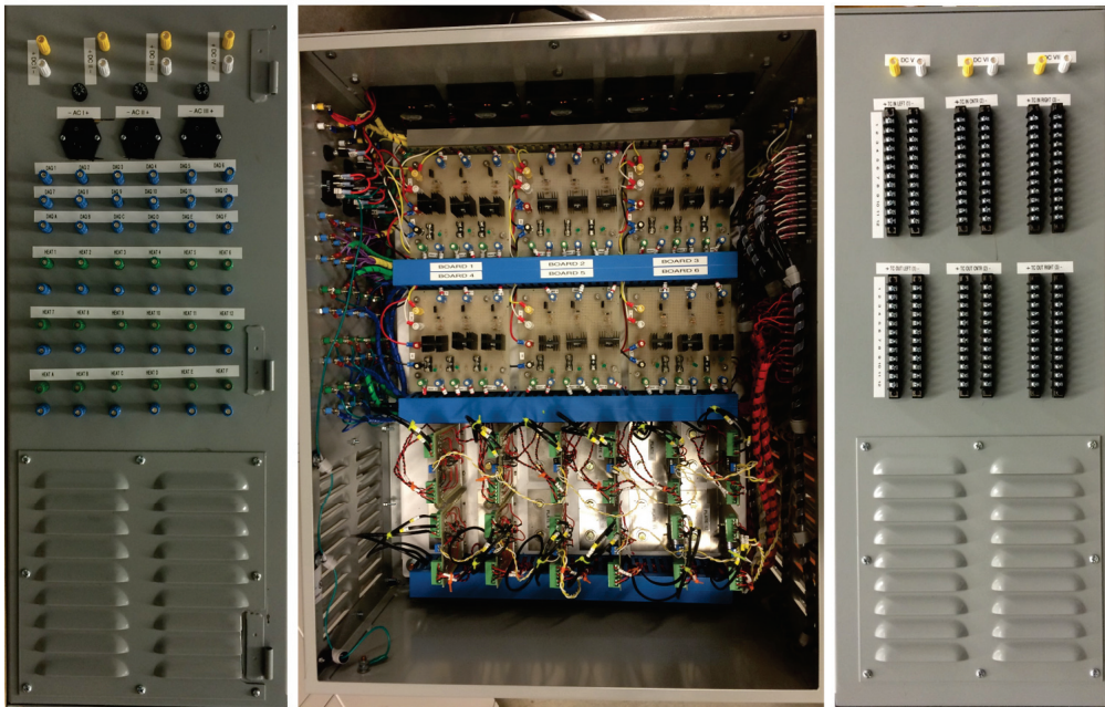
Figure 2.10: Top: the assembly process of the electronics in the enclosure box. Bottom: the final preview of the enclosure box before wiring the heaters and thermocouples.
