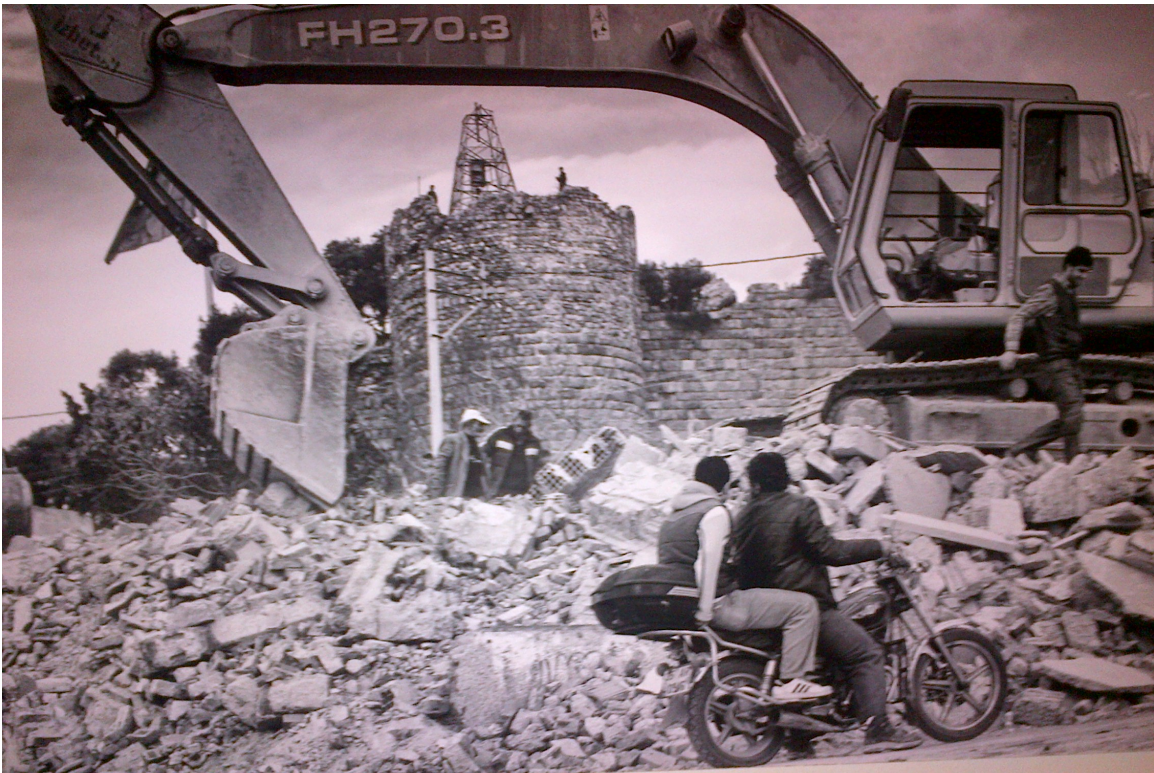
Photo IV: The Demolishment of Kadifekale Neighborhood, from Ozlem Tezcan, Serkan Colak and Sinan Kilic (2013, December 16). Kadifekale and Urban Tranformation
