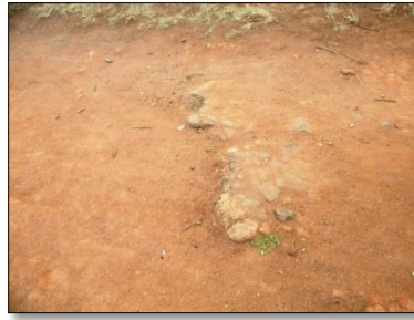
Figure 5.7: Evidence of daga flooring being eroded along the pathway
