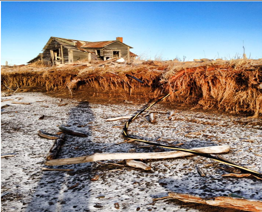
Figure 1.2 Shaktoolik: Old power house. Wire exposed in the old power house. Photo taken after the storm of November 9, 2013. Credit: Gloria Andrew
